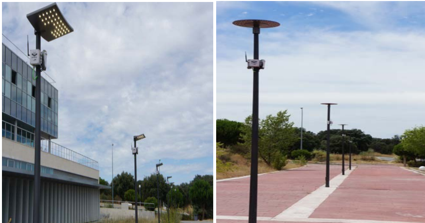
Figure 53. Low consumption street lamps installed on the Campus
