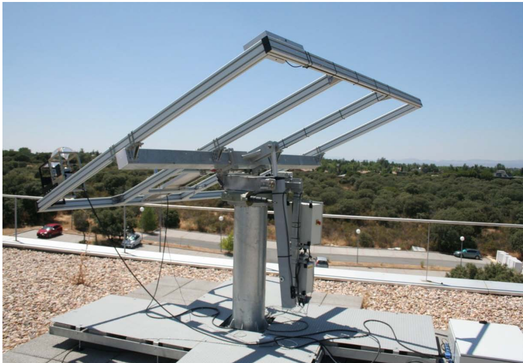
a) Cell, optic and array (model and “tracker installed on the terrace at CeDinT) of the de photovoltaic concentration pilot plant
