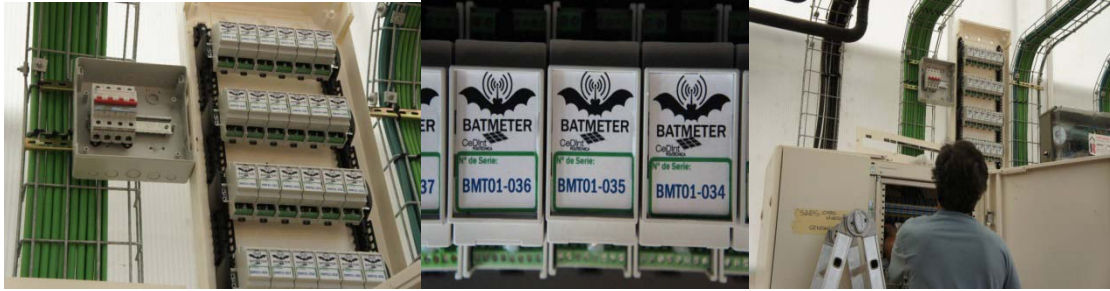
a) Modules for the measuring of consumption
